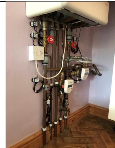
Pipework - post meter install
